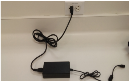
A/C Power Supply - Connected to wall outlet
